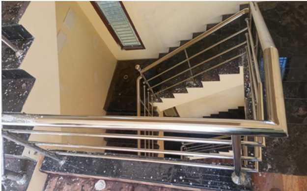
SS & MS STAIRCASE RAILING
